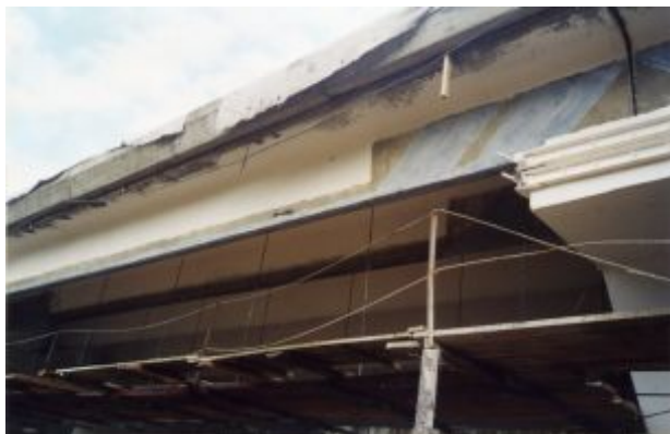
Picture 5 - Gluing of the canvases to the end sections of bridge girders through Kirzhach river (2002) (presentation of FSUE «ROSDORNII»)
